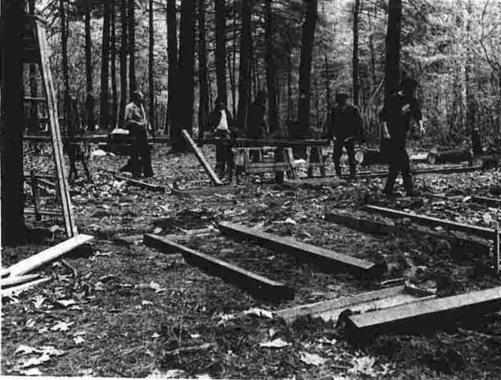
Jungle gym for Peoples Park Manchester Community College faculty members constructed a jungle gym for a People's Park, the Bicentennial project for the college campus last year. John Sutherland, assistant history professor (third from left) was chairman of MCC's bicentennial activities. (Herald photo by Dunn)
